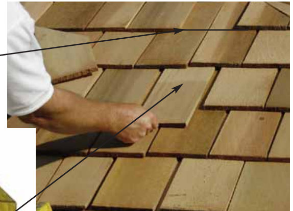
118. Slide in the next long Filler Shingle and attach as per Step 117 . Continue until top row. On top row, slide in Short Filler Shingle and attach with 3" screw into Mid Rafter. Important - Work around the gazebo making sure to slide in all Filler Shingles and attach Roof to Mid Rafter as per Step 117 .
