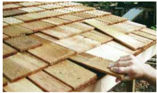
116. Next, time to install Filler Shingles to completely secure gazebo roofs and hide roof seams. Starting on bottom row of shingles, push a Long Filler Shingle (5 1/2" wide) underneath shingles directly above it until end is flush with bottom shingles.
